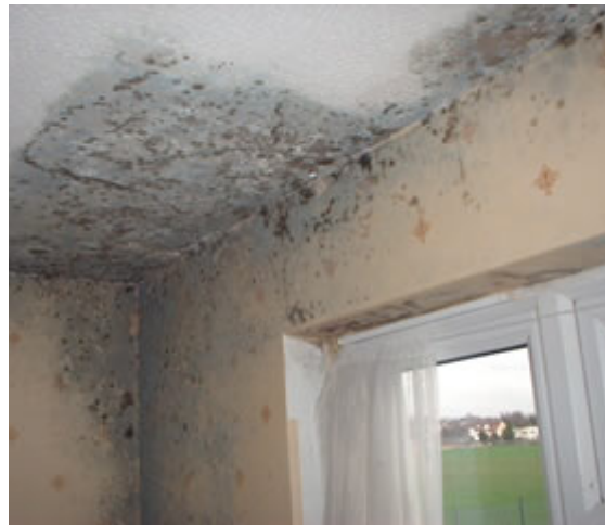
Figure 8: Indoor molds on walls and AC vents can cause increase spore content indoors
