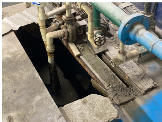
Figure 23: Dirty water accumulation in air compressor room
