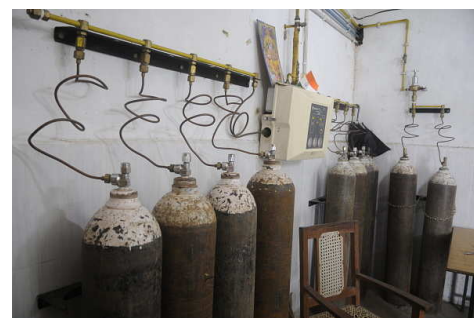
Figure 35: Cylinder manifold rooms are usually not well ventilated
