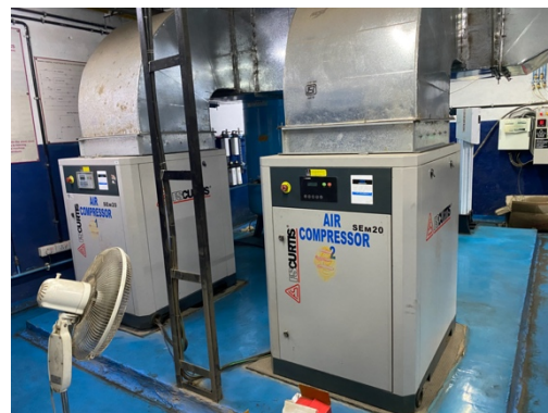
Figure 22: In house air compressor in a tertiary care center
