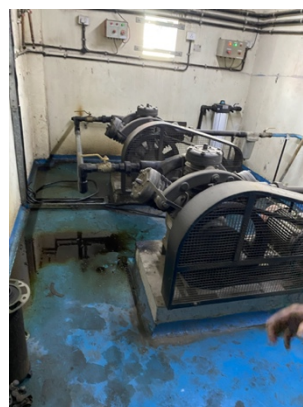
Figure 24: Unhygienic conditions near air compressor room
