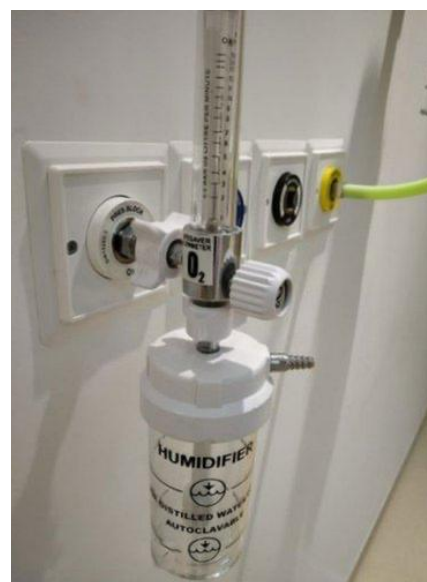
Figure 18: Humidifier must have a temperature regulator
